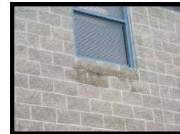
Left: water infiltrates through improperly detailed windows
