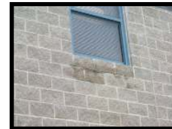
Left: water infiltrates through improperly detailed windows
